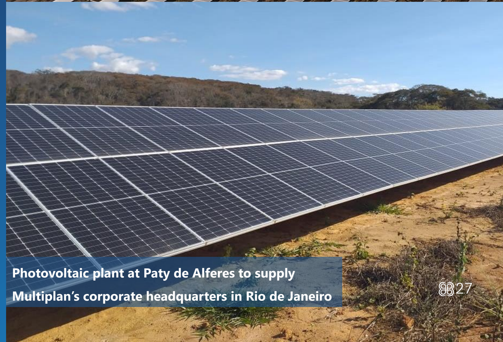
Photovoltaic plant in Minas Gerais to supply VillageMall
