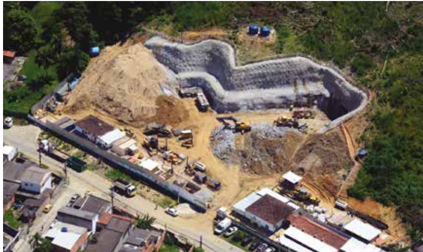
Works to modernize Campo Grande's road system, which received funding from BNDES Photo: João Luiz dos Anjos
