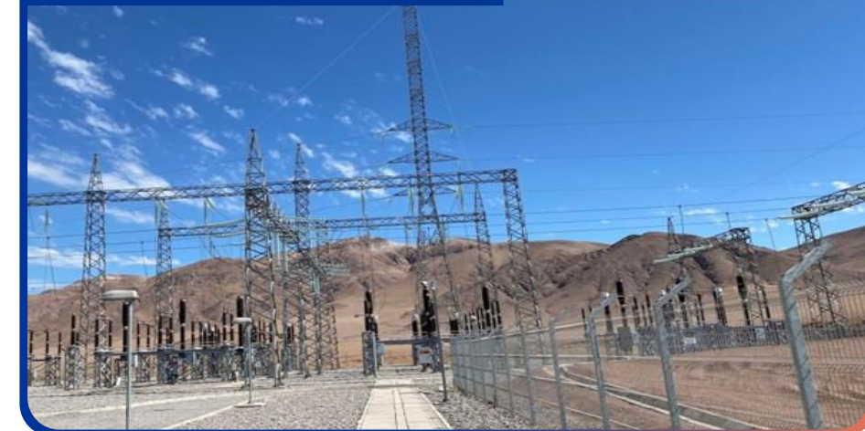
TecnoCAP – Transmission lines
