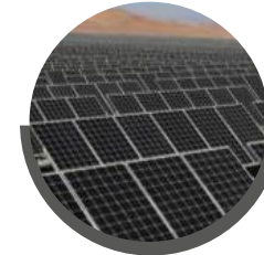
Structures for solar panels
