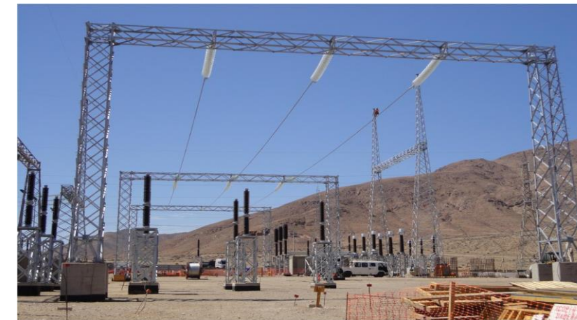
Power transmission line: Tecnocap
