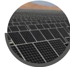
Structures for solar panels
