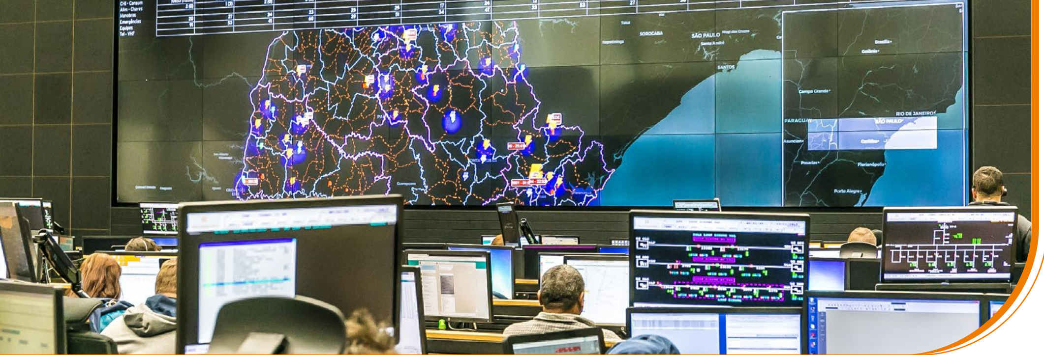
Integrated Power Distribution Center, in Curitiba-PR
