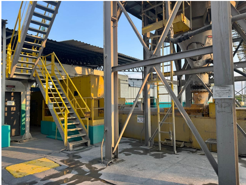
Figure 16-19: Xavantina paste fill plant, Piston Pump Duplex KSP 220XL + EHS 4500 (NX Gold, 2024)
