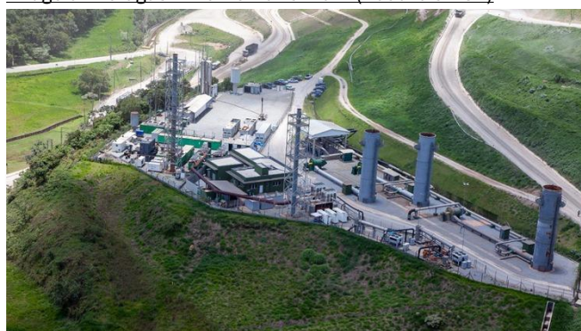
Image 9: Metagás – Biomethane Plant (Ecourbis – SP)
