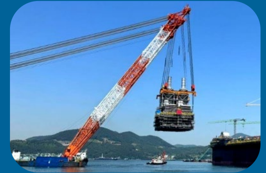
P-79 Completed the 5 modules executed in Brazil. Lifting of modules in progress
