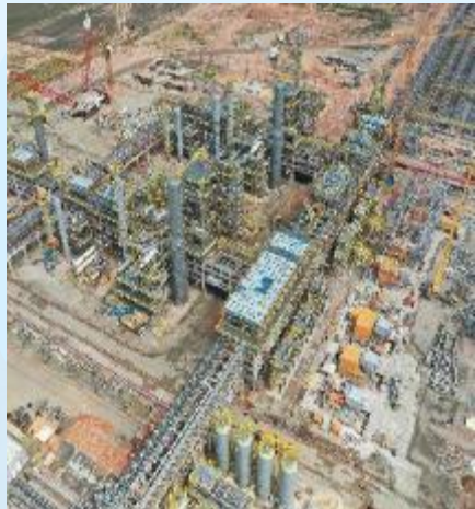
Gas processing plant Route 3
