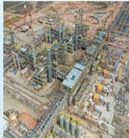
Gas processing plant Route 3
