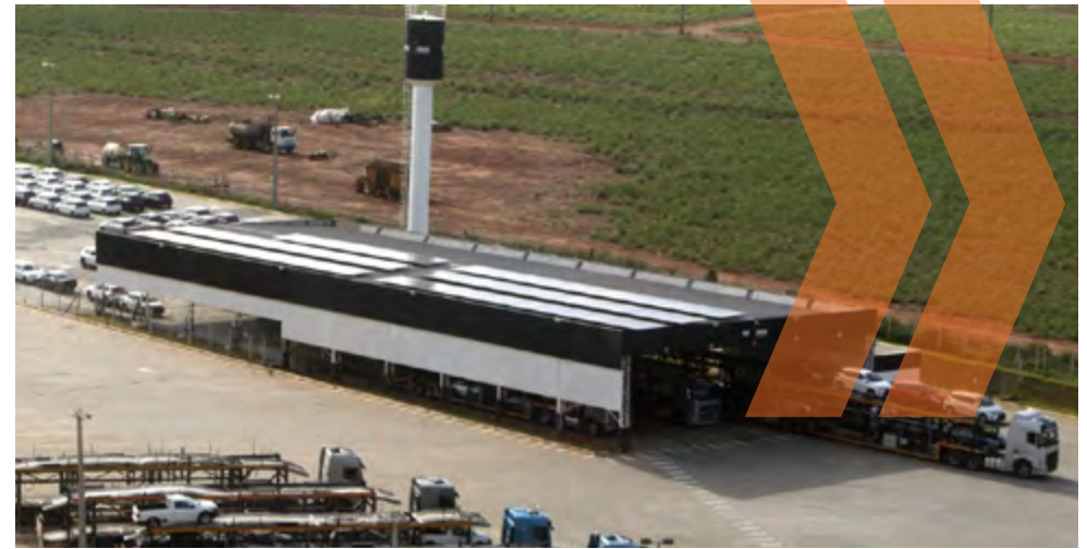
Photovoltaic plant operating at the Sorocaba unit
