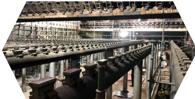
Plate oven 2 LTQ2 Initial Step– Revamp LTQ#2
