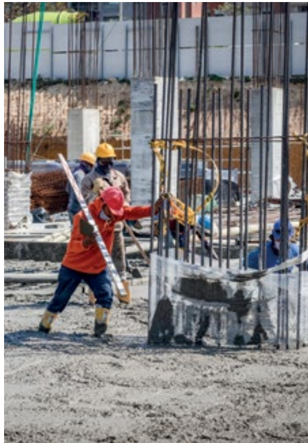
↑ Mass concrete pouring for the construction of the new Sura complex in Barranquilla, Colombia
