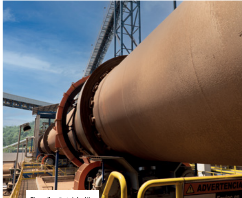
Thermally activated clay kiln Rioclaro Plant, Colombia Region.
