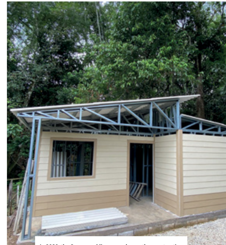
In 2020, the Casa para Mi program began the construction of the first rural housing pilot in La Danta, an area near our Rioclaro Plant, in Antioquia, Colombia.
