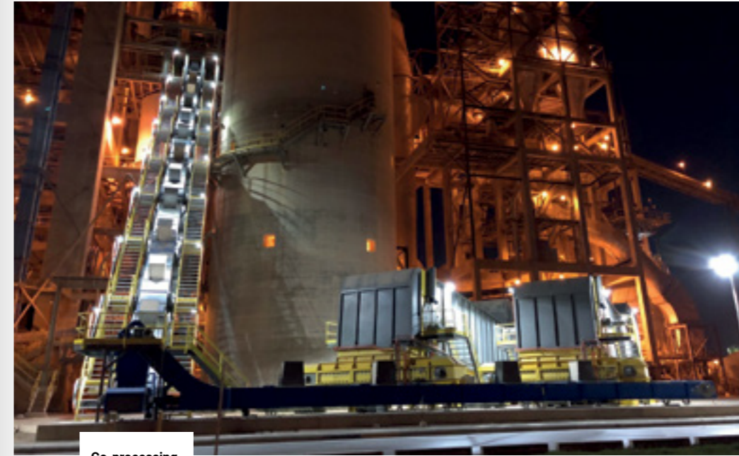
Co-processing in the Cartagena Plant; Colombia Region.
