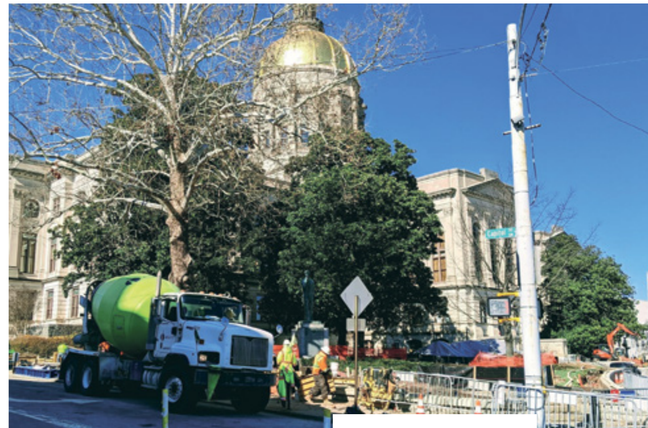
By pouring concrete into the Capitol Building in Atlanta, Georgia, we fuel development.
