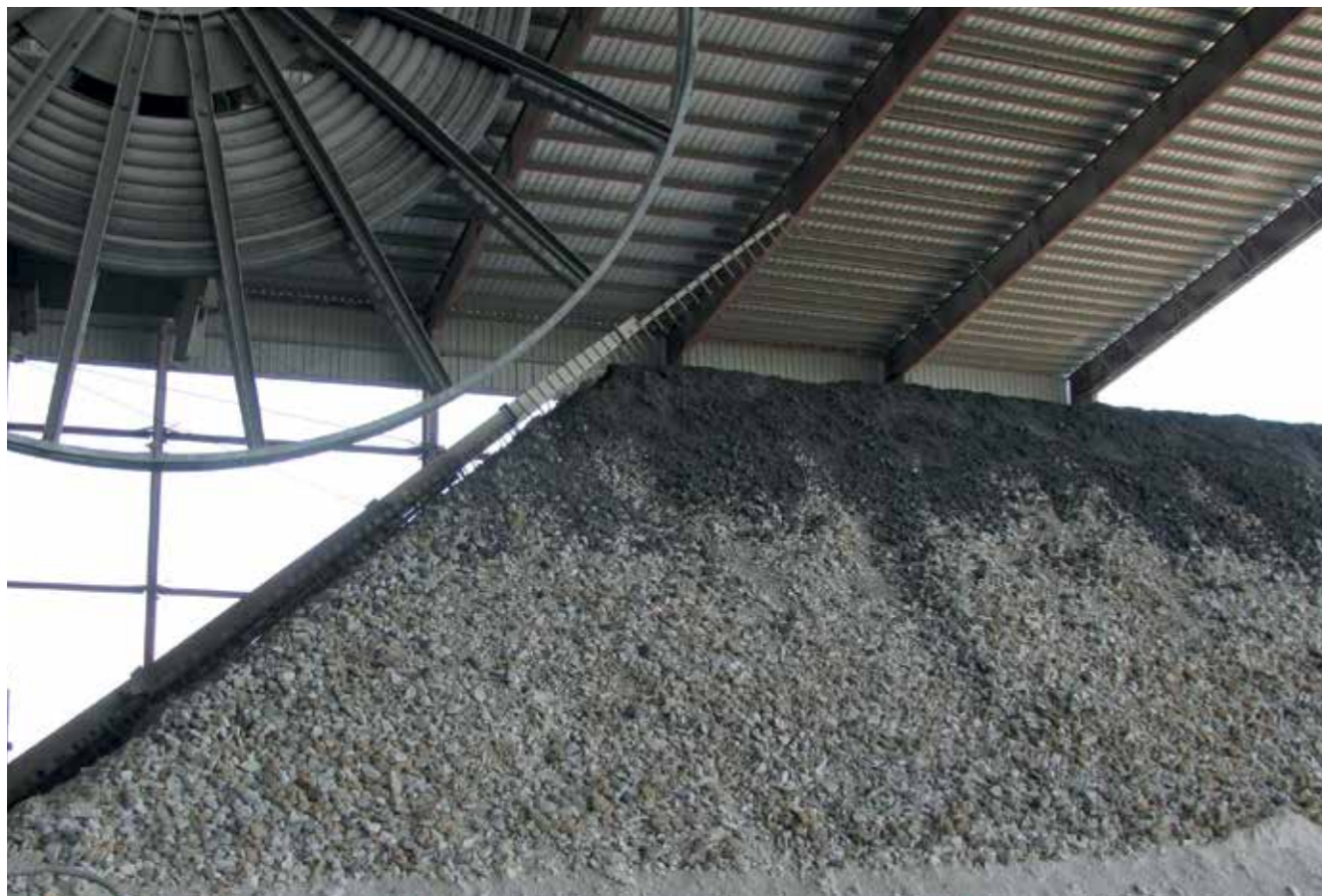
Homogenization system of raw materials fed to the clinkering furnace. Roberta Plant, USA
