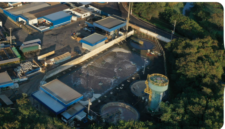
Effluent treatment plant, Cattle Unit, Lençóis Paulista/SP
