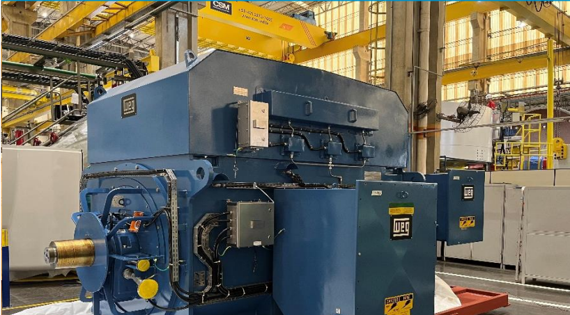
Carbon Capture Slip Ring Motors
