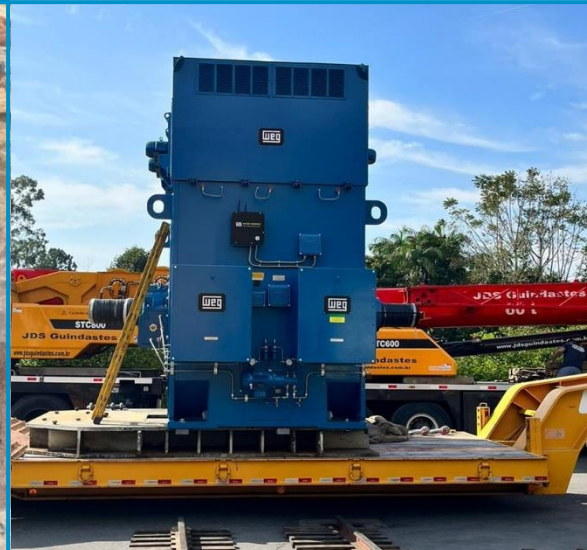
ARES Nevada Project 50MW/12.5 MWh
