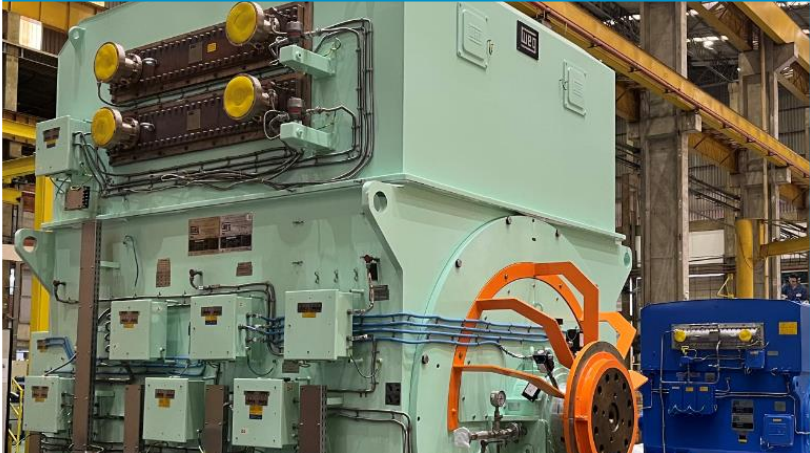
Generators Oil & Gas Offshore
