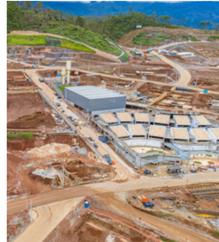
Works of the Resettlement of Bento Rodrigues, in Mariana (MG). Photo: Guilherme Guedes
