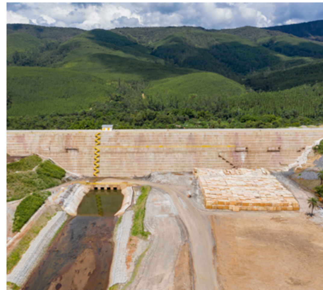
Implementation of the downstream containment (backup dam) of the Sul Superior Dam, in Barão de Cocais.
