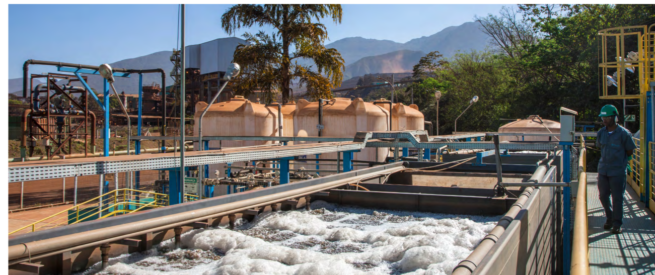
Alegria Mine effluent treatment plant – Minas Gerais, Brazil. Photo: Ricardo Teles
