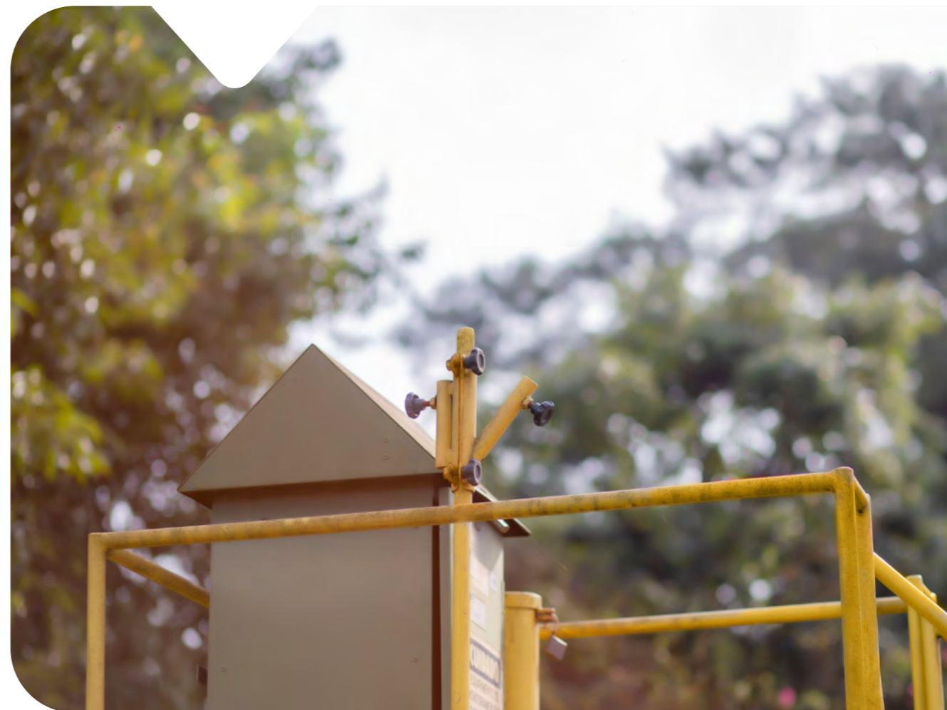
An air quality monitoring system
