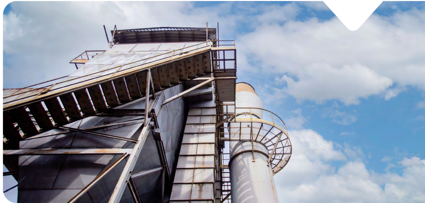
An air emissions control system
