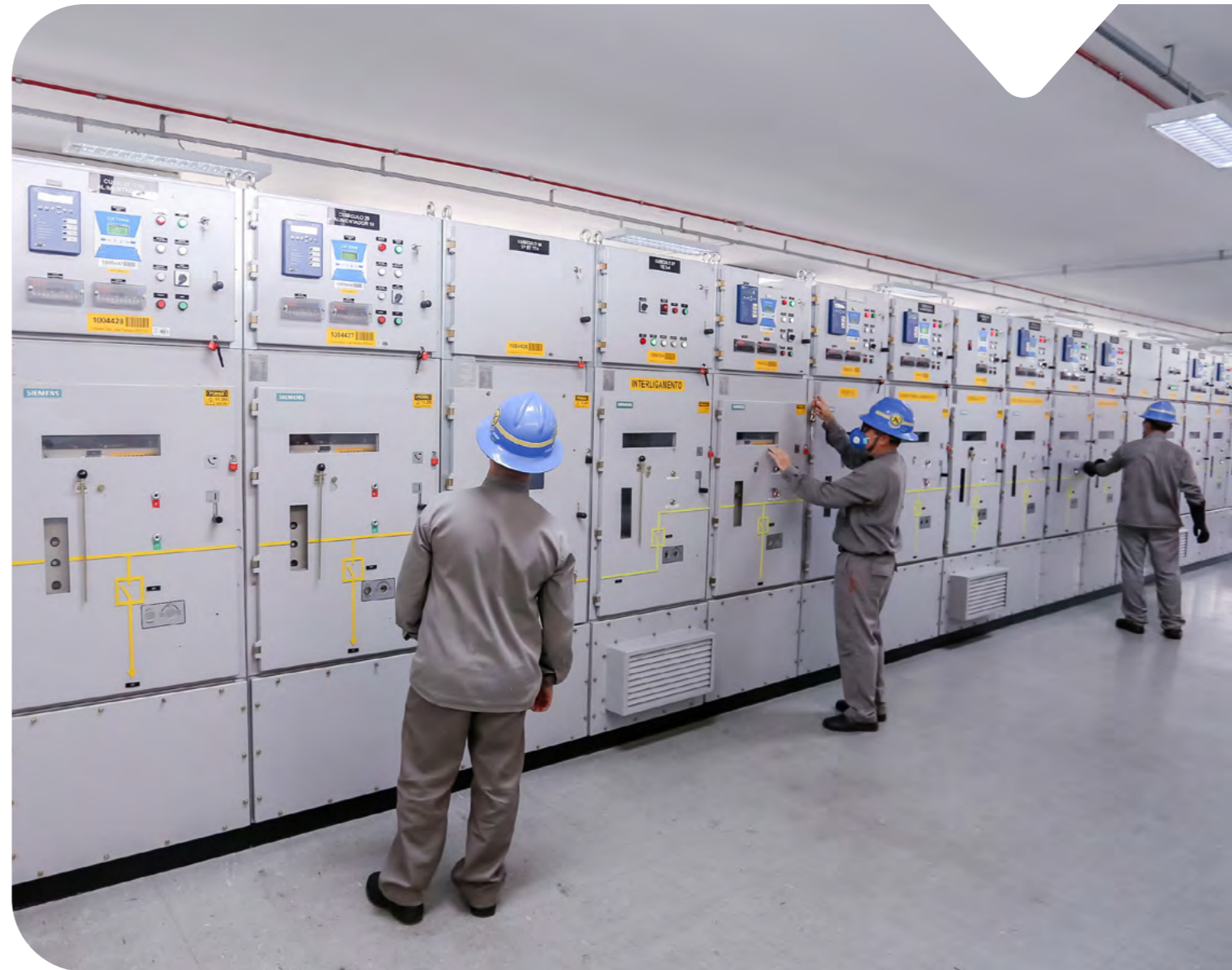
Members of the Energy Efficiency Group in a switchgear room
