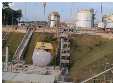
GTU: Knockout drum assembly
