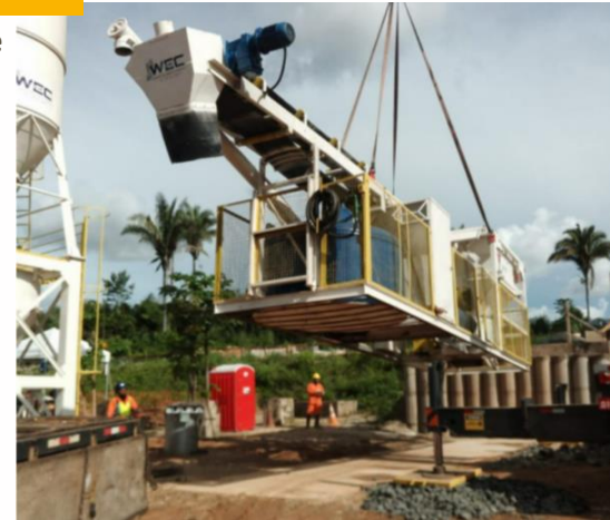
Silo and Plant installed on site
