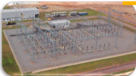
Jaguaririca Substation 100% operational
