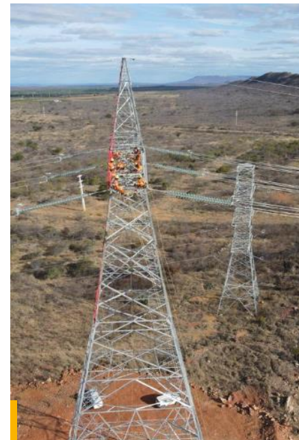
500 kV Transmission Line
