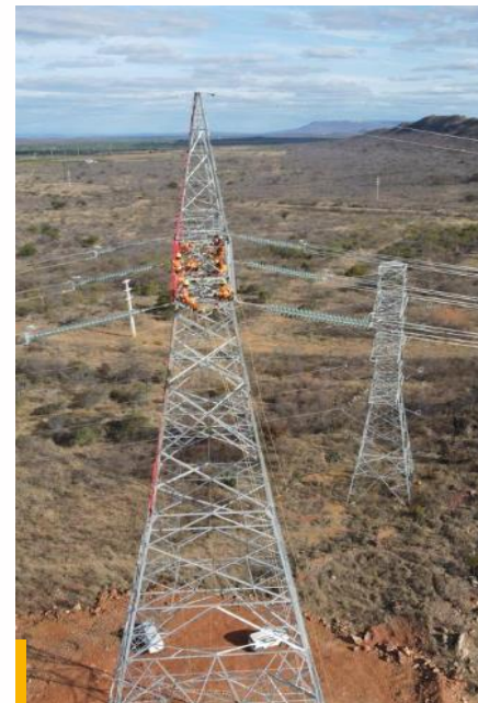
500 kV Transmission Line
