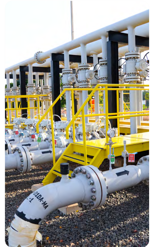
Gas Pipelines in the Parnaiba Complex
