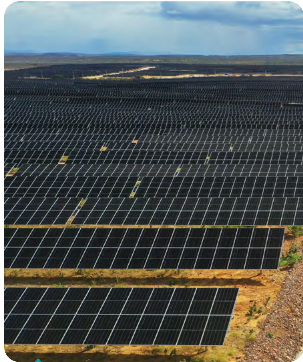
Futura I Solar Complex
