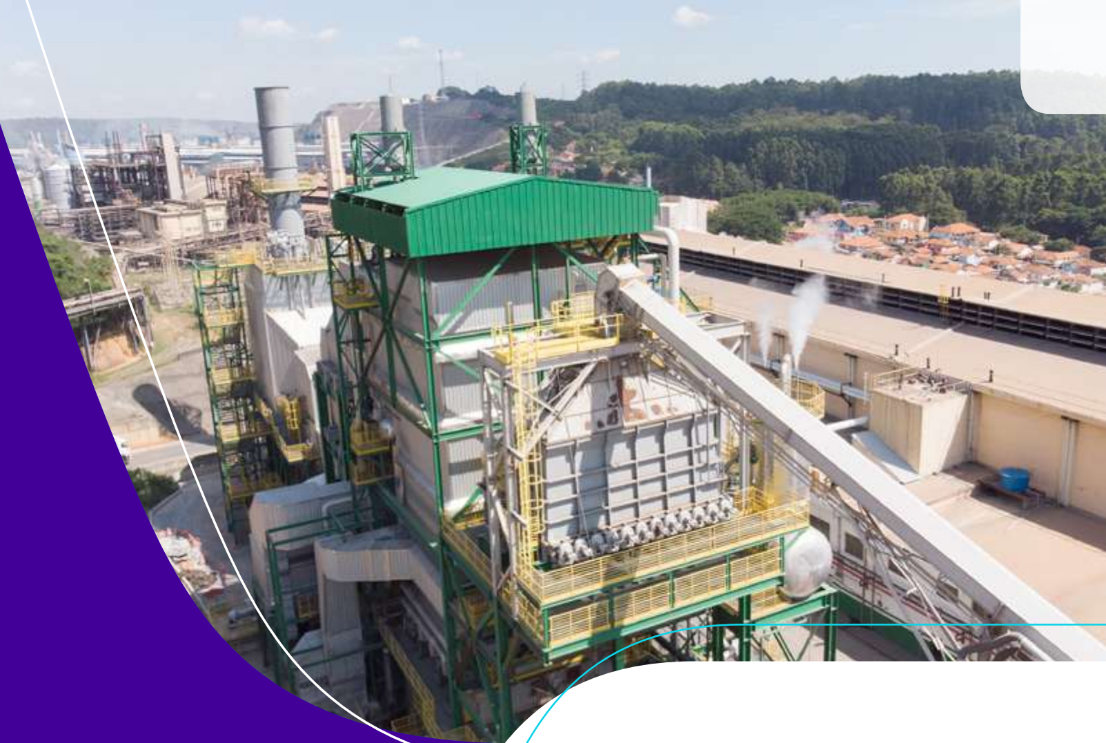
A biomass boiler in the Refinery at Alumínio Plant (SP)
