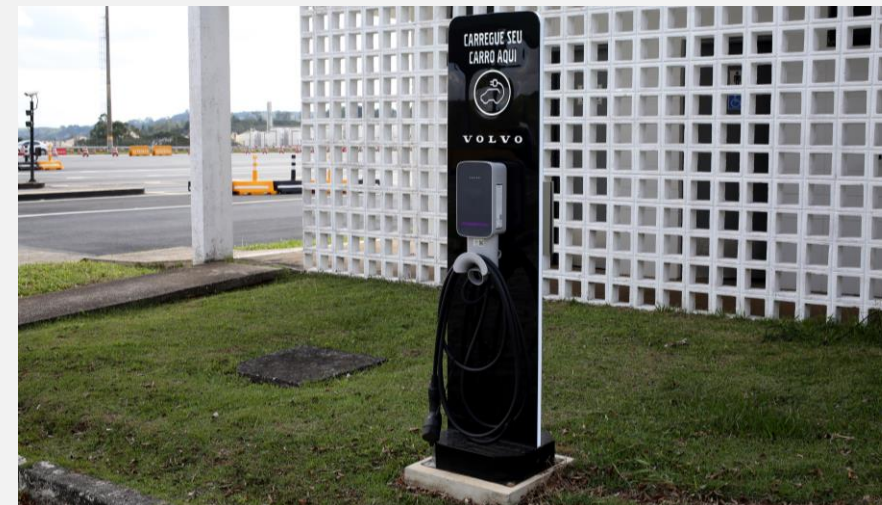
Electric charger installed at an EcoRodovias Group unit
