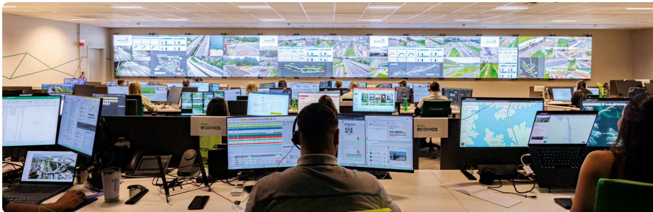
Operational Control Center SP Nucleus
