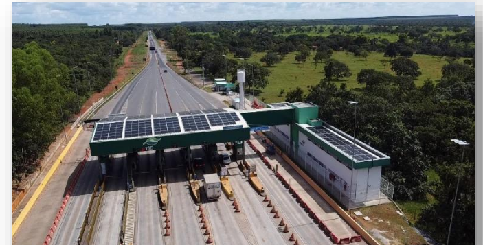
Photovoltaic panels installed at Eco135 toll plaza
