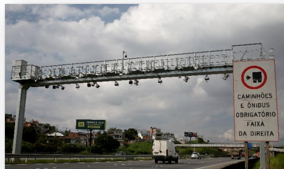
Free Flow gantry in test at Ecopistas
