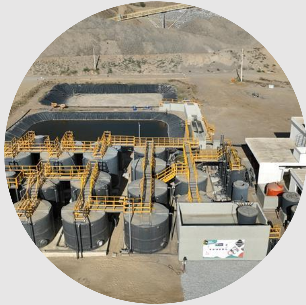
Sewage Treatment Plant Borborema, RN
