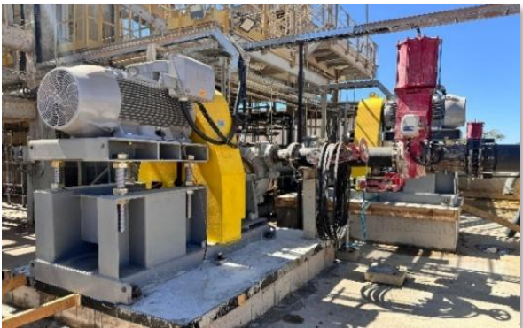
New tailings pumping system
