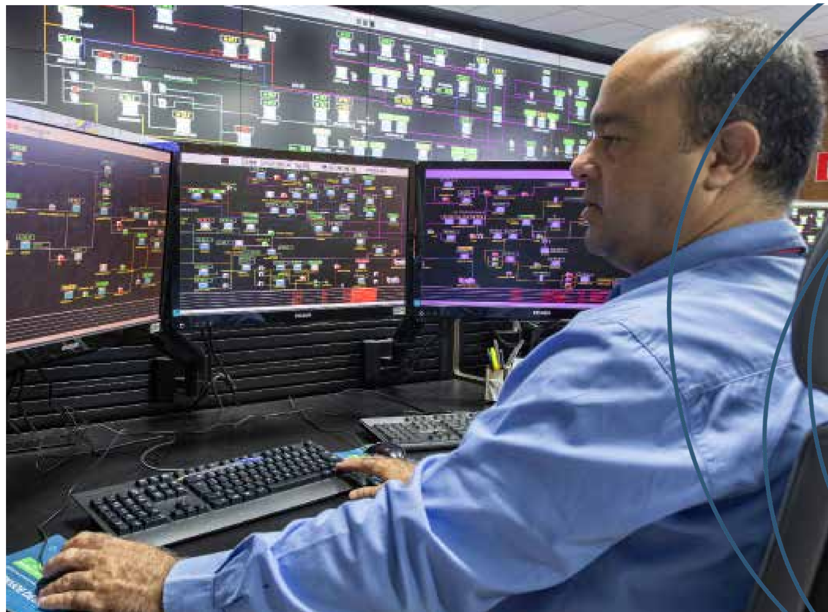
Copasa, Control Room
