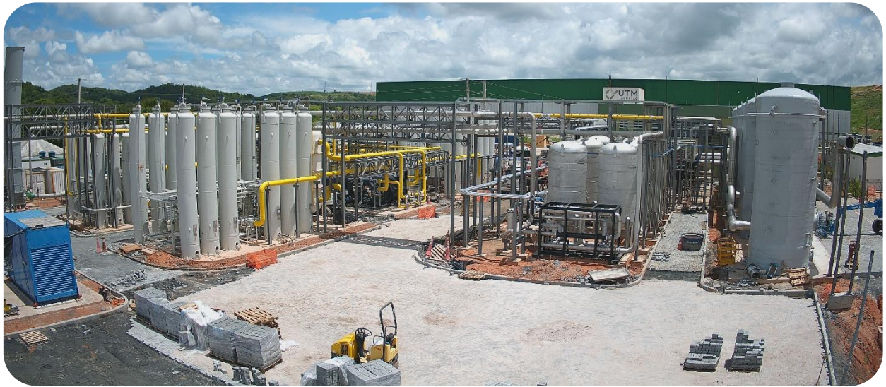
Photo: Construction site for the implementation of the biomethane project in Paulínia in March 2025.
