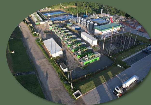
Biometano – Jabotão dos Guararapes Expected Start Operations: 2H25
