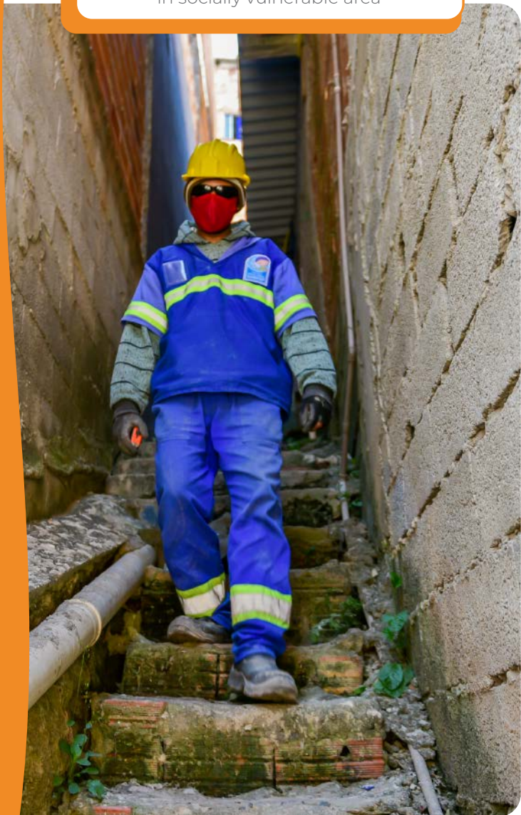
Employee in action on water supply regularization work in socially vulnerable area
