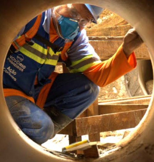
Employee at work for the expansion of the sewage collection and treatment structure in Greater São Paulo
