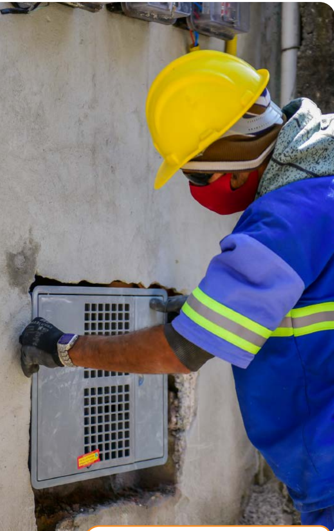
Works to regularize the water supply system in the Jardim Savoyzinho neighborhood, East São Paulo city
