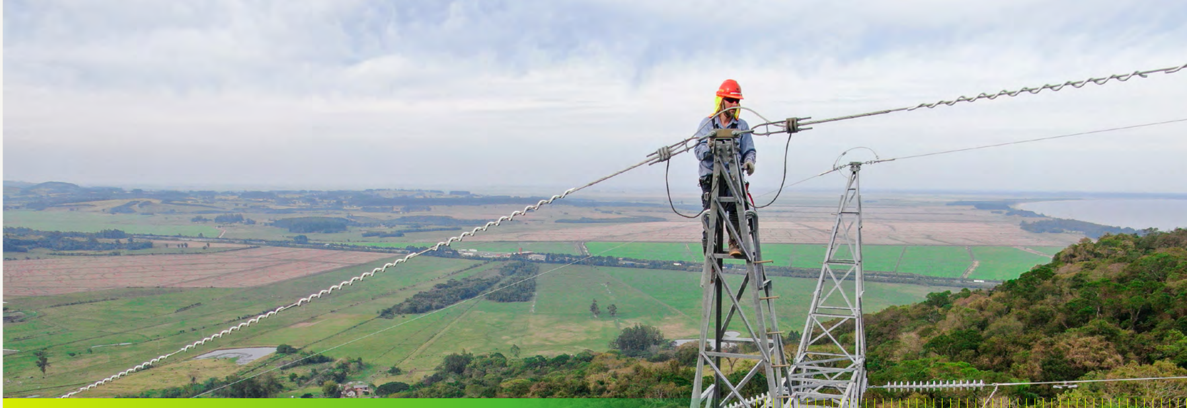
Maintenance of cables in a tower on the Atlântida 2 transmission line - Gravataí 3 - Photo: Marcelo Camargo Constante
