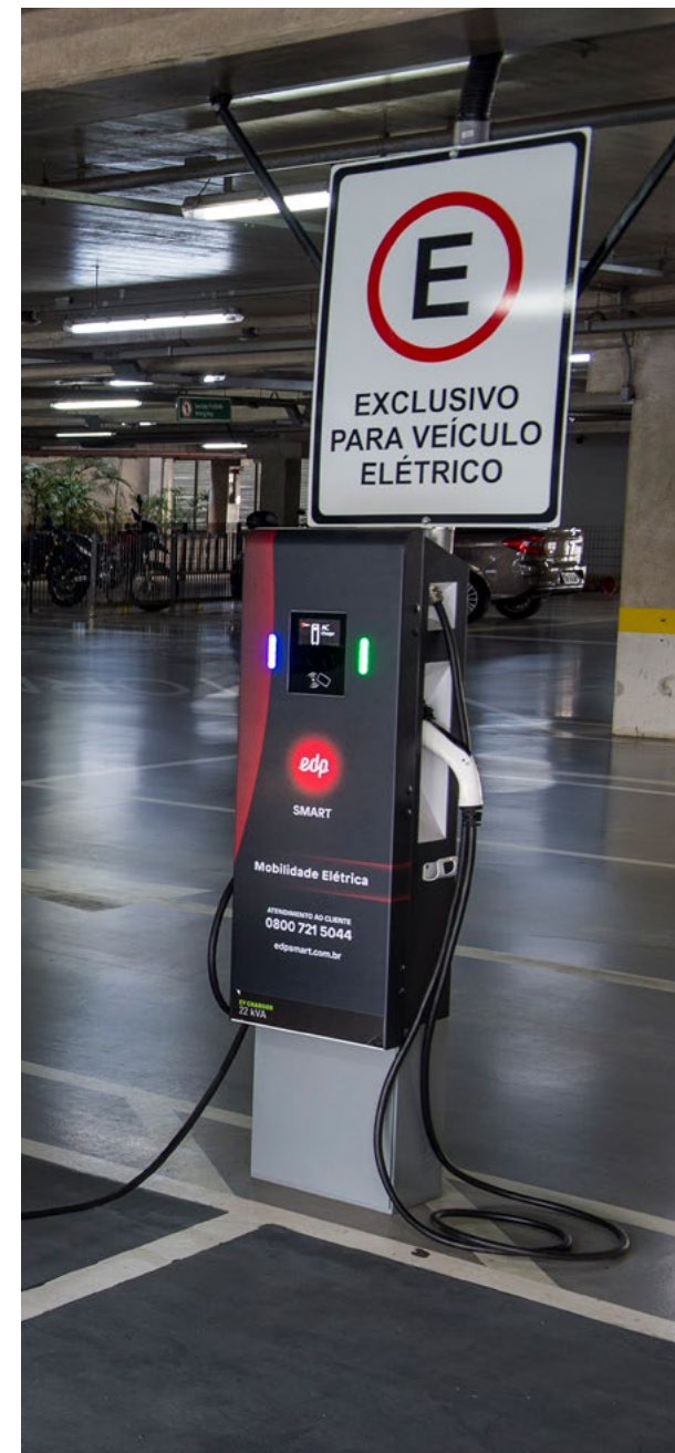
Electric vehicle charger.
