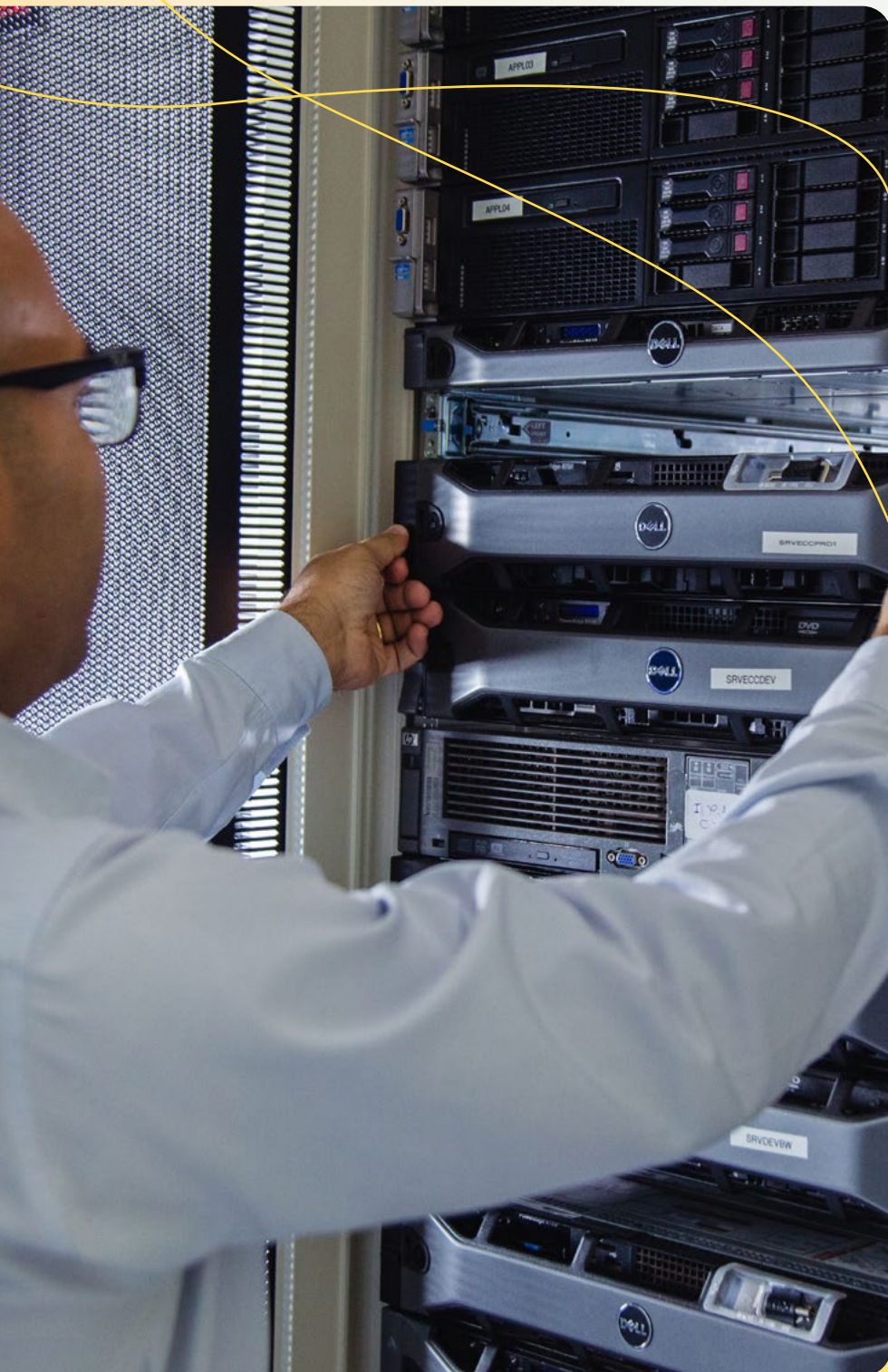
Data Center – Itumbiara (GO)
